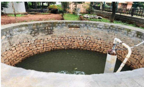
Open Recharge Well
