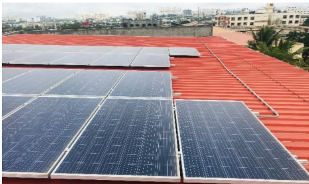
Solar PV system
