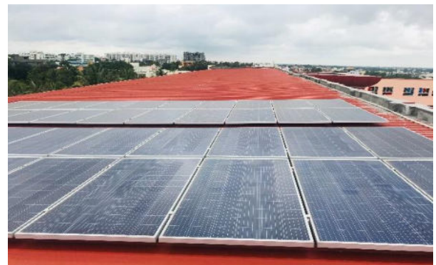
Solar PV system
